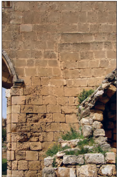
Figure 20. Hagios Georgios, Southern Wall, Vertical Joint at the West End of Hagios Epiphanius – Thomas Kaffenberger
